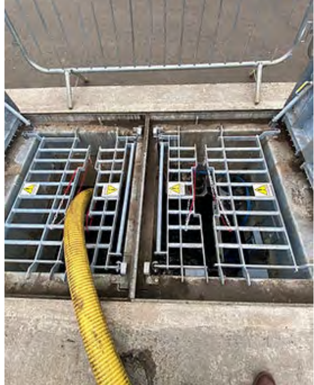
Example of a pumping station
